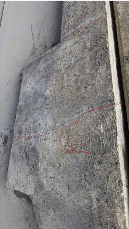
DEFECT 31: 2-Full Width Transverse Hairline w/Efflo.
