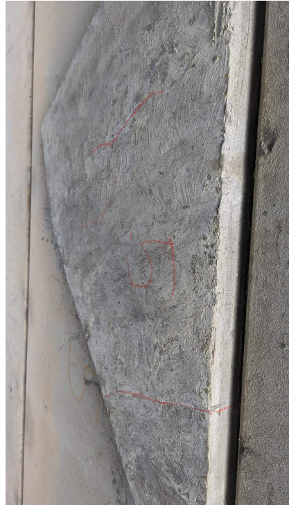
DEFECT 5: 2-18" Long Transverse Hairline Cracks
