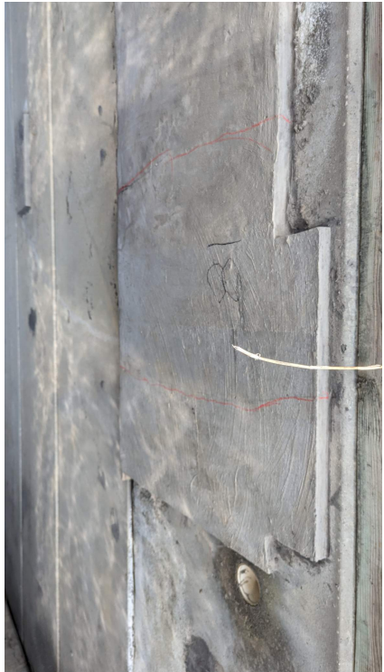
DEFECT 18: 2-Full Width Transverse Hairline to 1/32" Cracks
