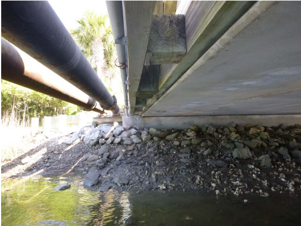
Visible panel repairs
