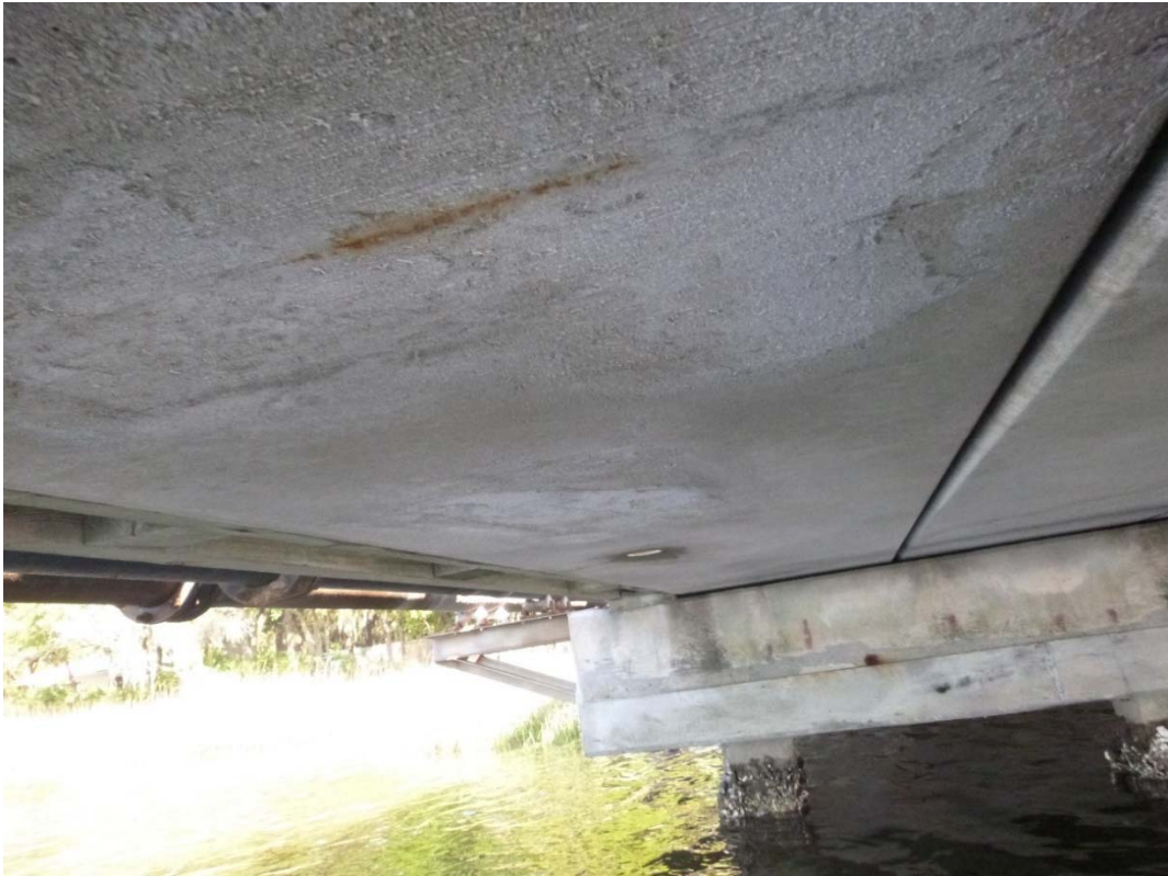
Leaching rust stains from bottom of stirrups bars
